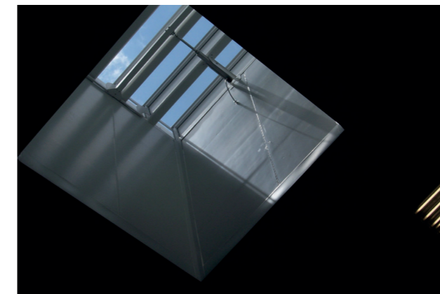
Brakel® Eura ventilators above the fans
